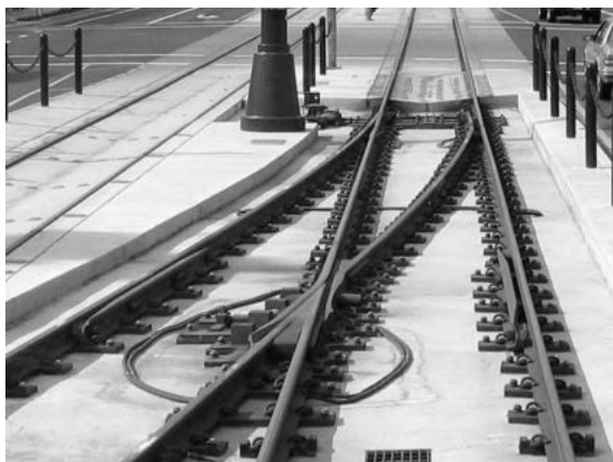
Photo 6.22 Modern rail switch with elastic points (Courtesy of James Aslaksen)
